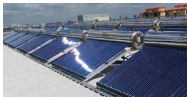
Roof Solar Panel
