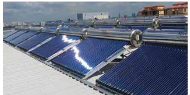
Roof Solar Panel
