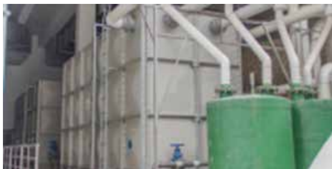
Rain Water Harvesting
