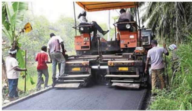
Useful material: A test road being built using cup lump-modified bitumen designed by Malaysian Rubber Board scientists in February 2020. — Malaysian Rubber Board
